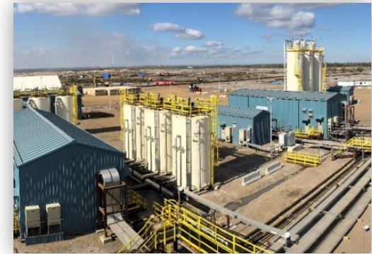
Waste water treatment plant
